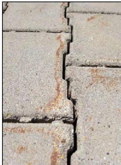
Rust marks from steel snow blades
