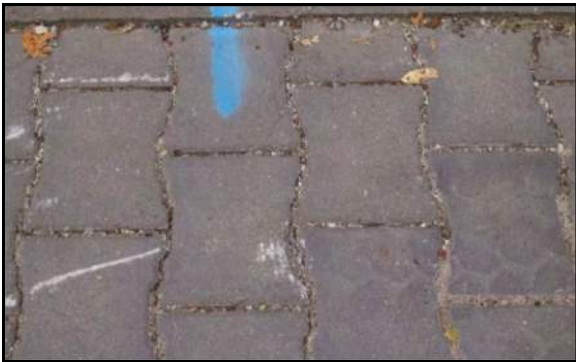
Photo 1 – PaveDrain in need of cleaning
