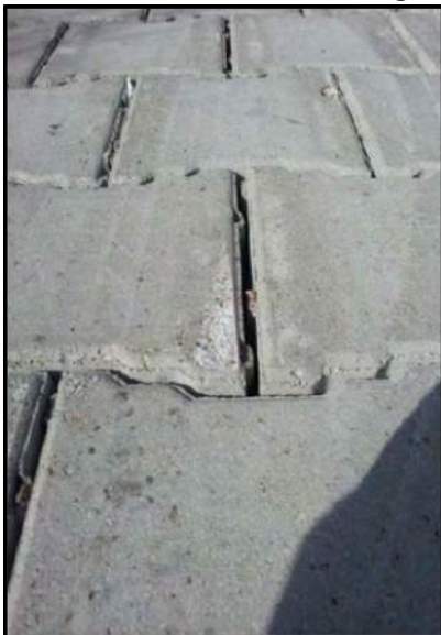
Steel Snow Plow Damage
